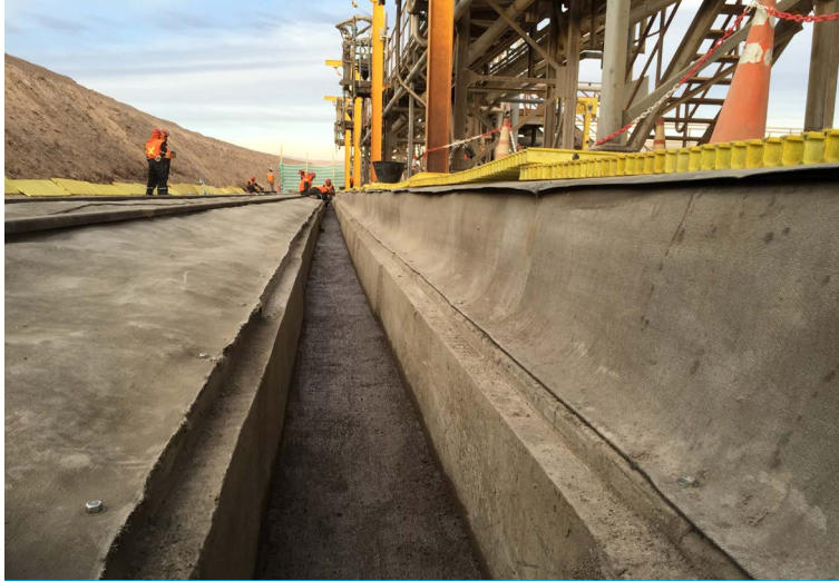
CC screwed to pre-cast concrete ditch
