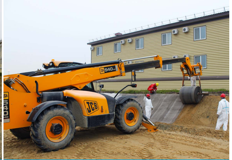
CC8™ bulk rolls were unrolled across the ditch and into anchor trenches
