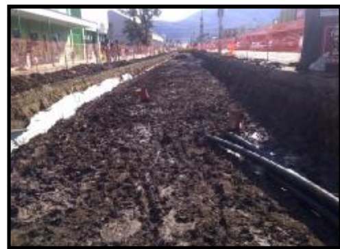
Waterlogged box cut
