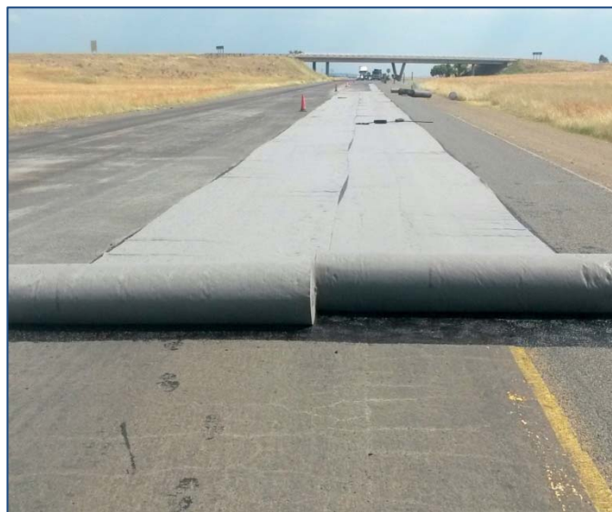
The road surface had been cracking and required repair
