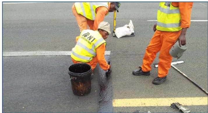
A bitumen emulsion is applied to the road surface before applying Sealmac ® strips
