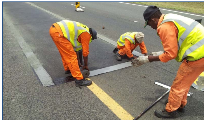
Sealmac ® strips are rolled out over the tack coat and any creases removed by squeegee
