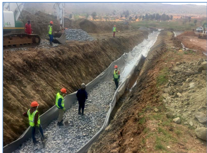
With sides lifted, RockGrid® PC encapsulates a layer of dump rock to serve as a reinforced base for stormwater pipes
