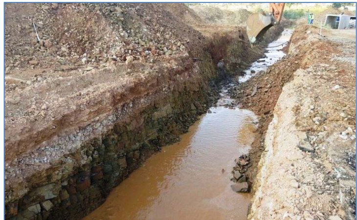
The low bearing capacity soil proved problematic for heavy stormwater pipes
