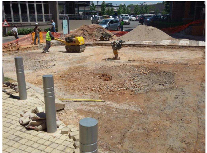
The roadbed was rolled to provide a flat surface to lay the TriAx geogrid.
