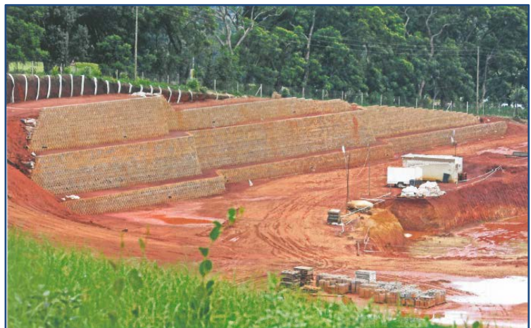
Retaining wall under construction at the new International Convention Centre and five star resort.
