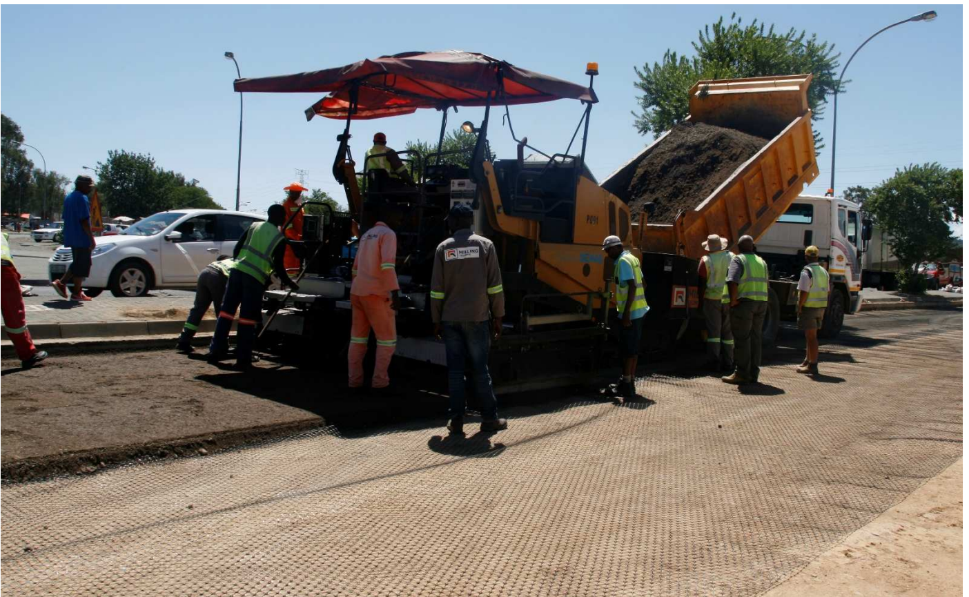
Foamed bitumen emulsion treated base material being spread by a paver directly onto TriAx Geogrids
