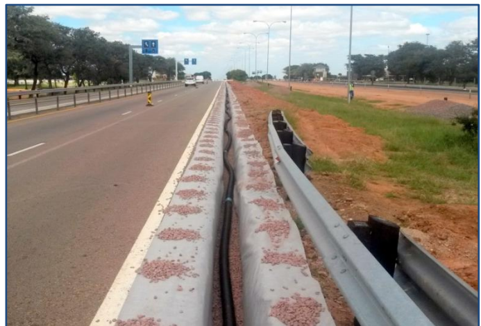
bidim ® and Flo-pipe drainage system used to channel excess water.
