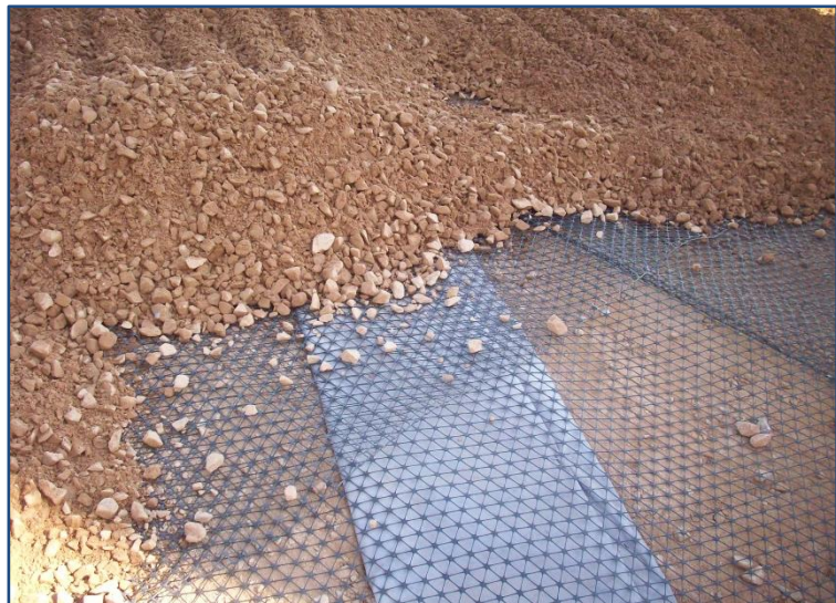
Kusile loading platform - compacted gravel covers the TriAx™ which is placed on top of compacted in situ soil.
