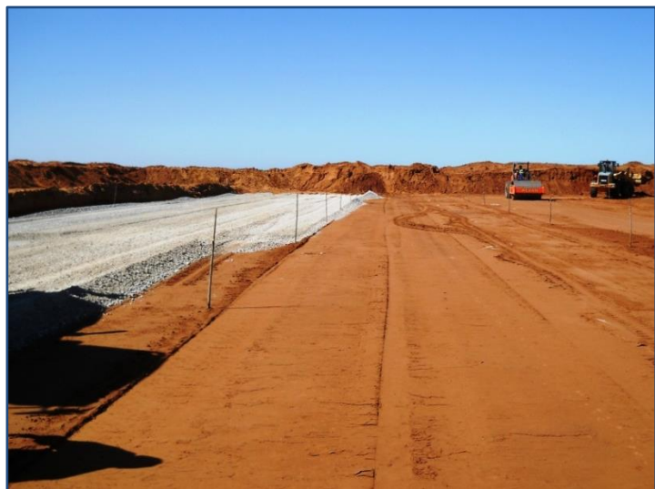
Sandy soil road with inherently low CBR qualities at Sere Wind Farm.
