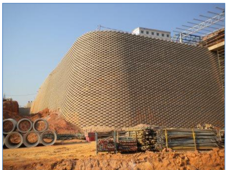
The 140m long, 15m high retaining wall which will support the new multi-level Watercrest Mall
