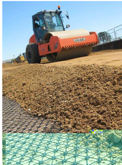
Right: Tensor TriAx geogrid placed on formation in lieu of ground replacement
