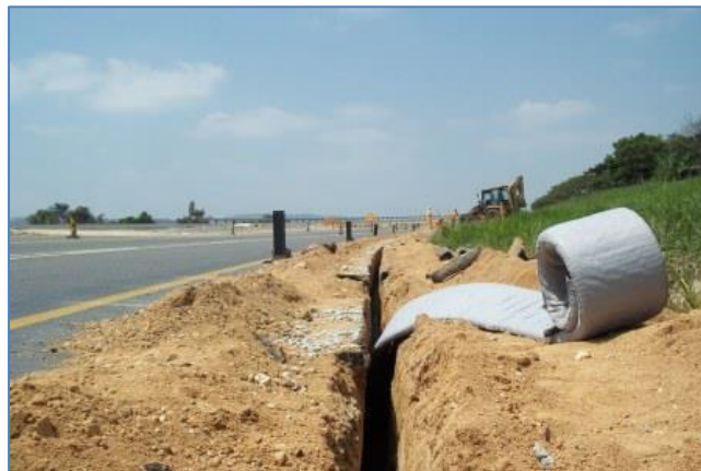
Megaflo™ 150 panel drain covered in a bidim® sock is laid into the narrow trench
