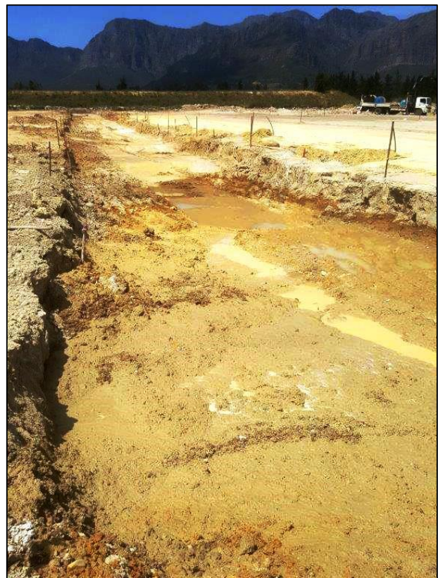
Main Access Road: Unsuitable insitu material
