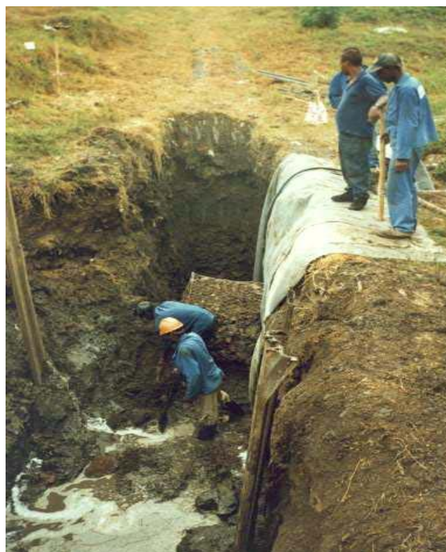
The Enviromat X1000 was pegged on the surface and suspended into the
