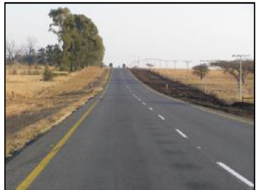
Km 32.200 – Sealgrid performance, July 2008. Note cracks have not reappeared
