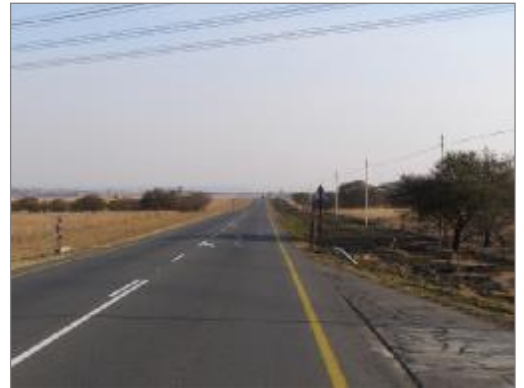
Km 16.28 – GlasGrid®/Sealmac® performance, July 2008. Note reappearance of cracks beyond culvert, outside area of geosynthetic repair
