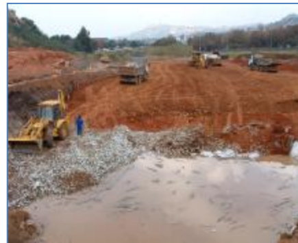
The sub-grade material - insufficient load bearing capacity
