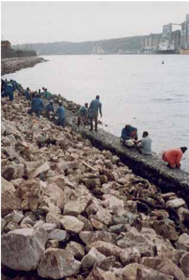
This photo clearly shows the gabion toe wall and the rip rap covering the Kaymat U44 .
