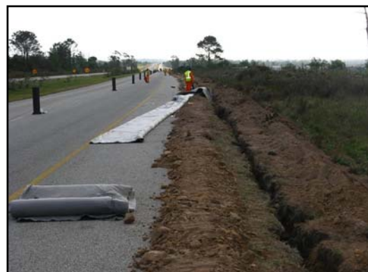
Installation of Flo-Drain into the ditch before being backfilled with river sand
